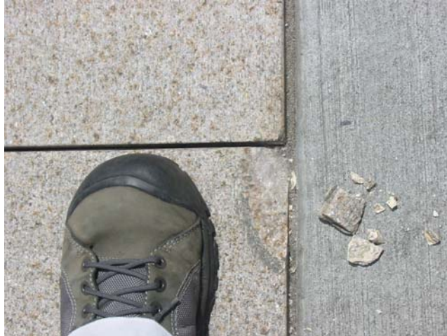
Figure 5 – Spalling of the festival traffic pavers
